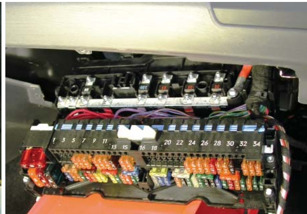
E83 fuse Panel behind Glove Box
